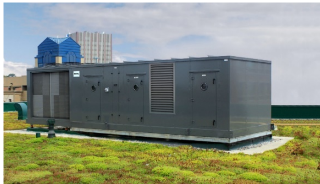
Air handling unit
